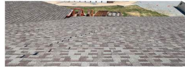
* The previous installation on roof area 2 also failed to follow the required "step-down" installation method. As seen in the picture above, the shingle seams fall >4" from each other. This is a very common mistake found on
