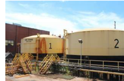
Ferric Chloride Storage and Containment Area
