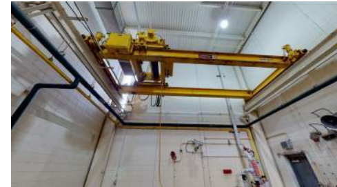
Coroded building crane from failed HVAC system
