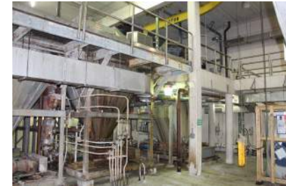
Primary Circular Scum House, Inside
