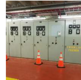
Representative Switchgear to be Replaced under CIP 111001
