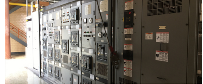
Service Building Electrical Substation
