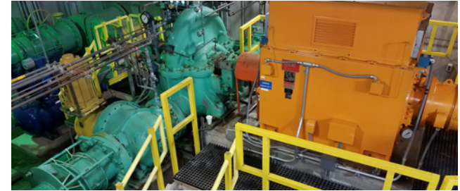
Joy Road Pumping Station
