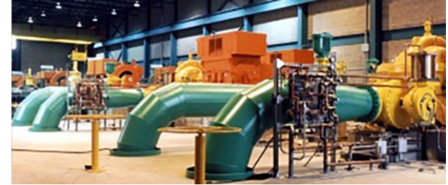
Franklin Pumping Station
