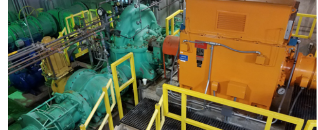
Joy Road Pumping Station
