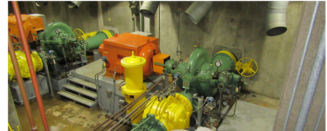
Adams Road Pumping Station
