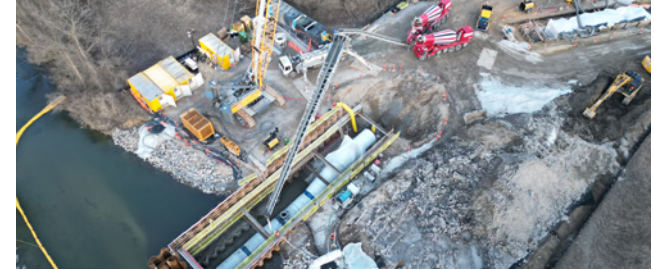
96-inch Water Transmission Main
