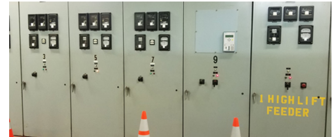
Lake Huron Water Treatment Plant
