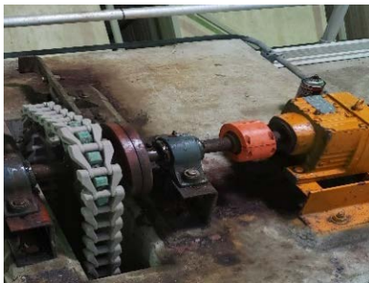
Sludge collector motor & drive chain
