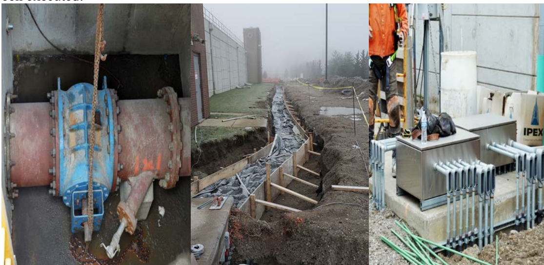
New Drain Valve # 3
