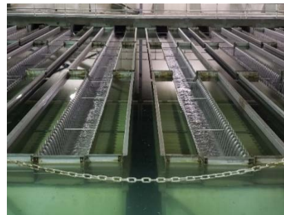
Sed Basin 1A back in service
