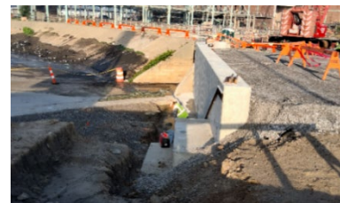
Ash Lagoon Concrete Form at the beginning and end of the month
