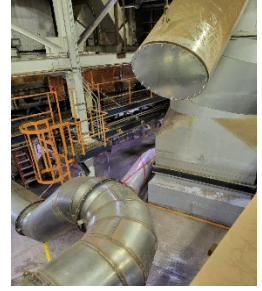
Blind flange where the exhaust used to route and new exhaust piping at the bottom of the image
