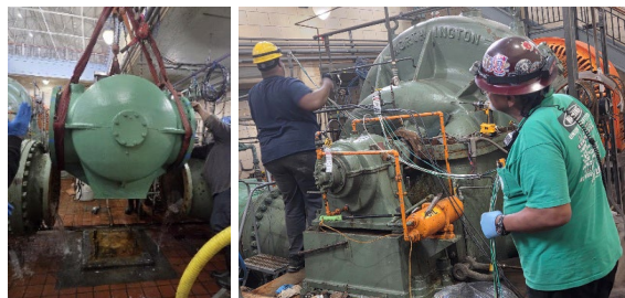
Maintenance Technicians and Electricians
