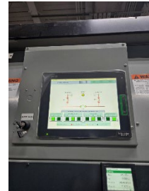
New PLC/HMI installed in EB-26
