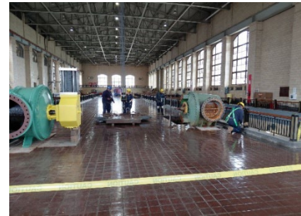
High-Lift Pump No. 22
