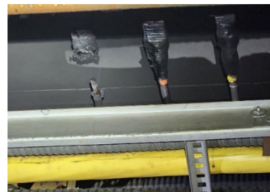
Motor connection damage
