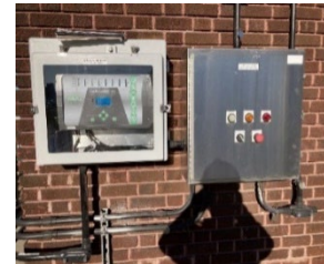
Gas Detection Controller and Alarm Panel
