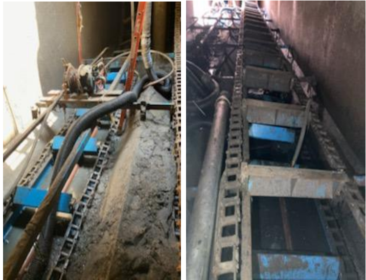
Grit channel at Pump Station 1 in the process of having its chain repaired
