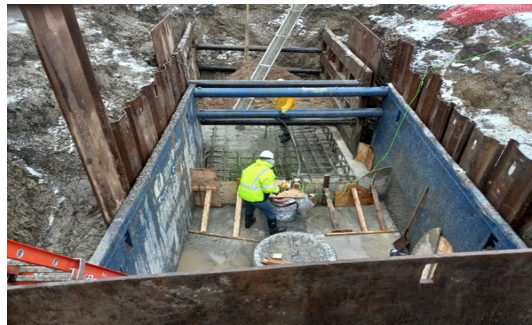
Pouring concrete for thrust block on the Garland-Charlevoix water main in preparation for linestop installation
