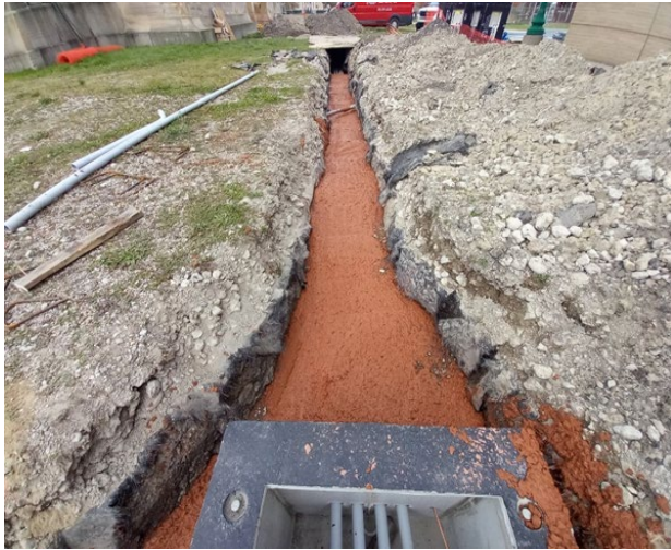
Electrical duct bank and handhole supplying power and instrumentation lines to future valve vaults
