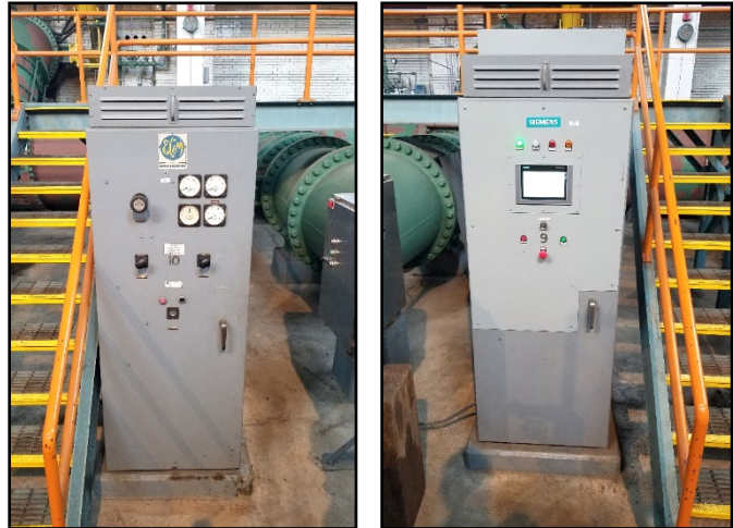
Existing Exciter Cabinet
