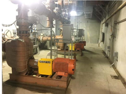
Residuals Equalization Basin Pumps
