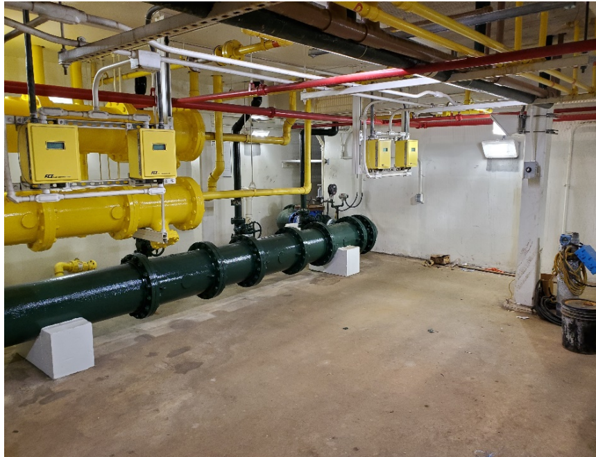
Newly repainted process piping and new lighting fixtures in dechlorination basement
