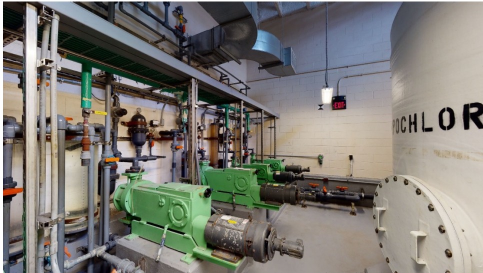
St. Aubin Chemical Feed Room
