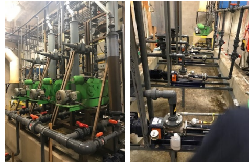
Old Metering Pumps
