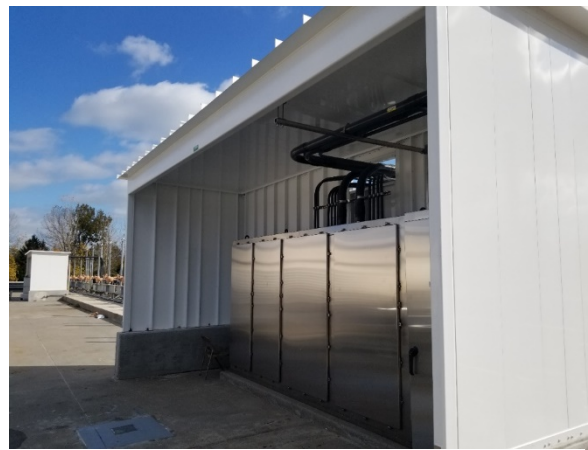
Shelter over Electrical/Communication Cabinets at Conner Creek CSO Basin
