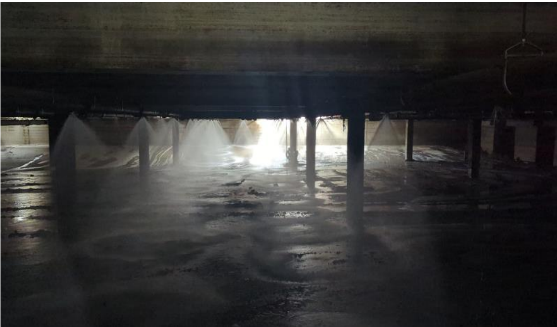
Existing Flushing System
