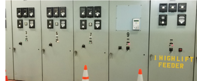
Lake Huron Water Treatment Plant
