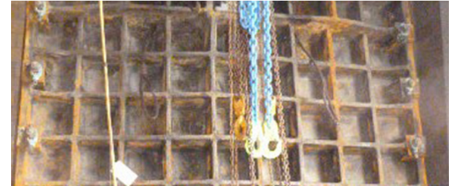
Sedimentation Basin Sluice Gates
