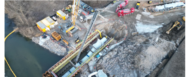
96-inch Water Transmission Main
