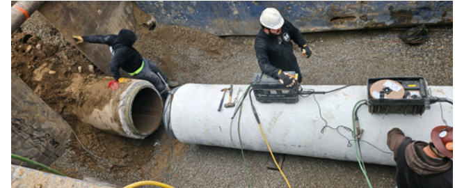
Transmission System Valve
