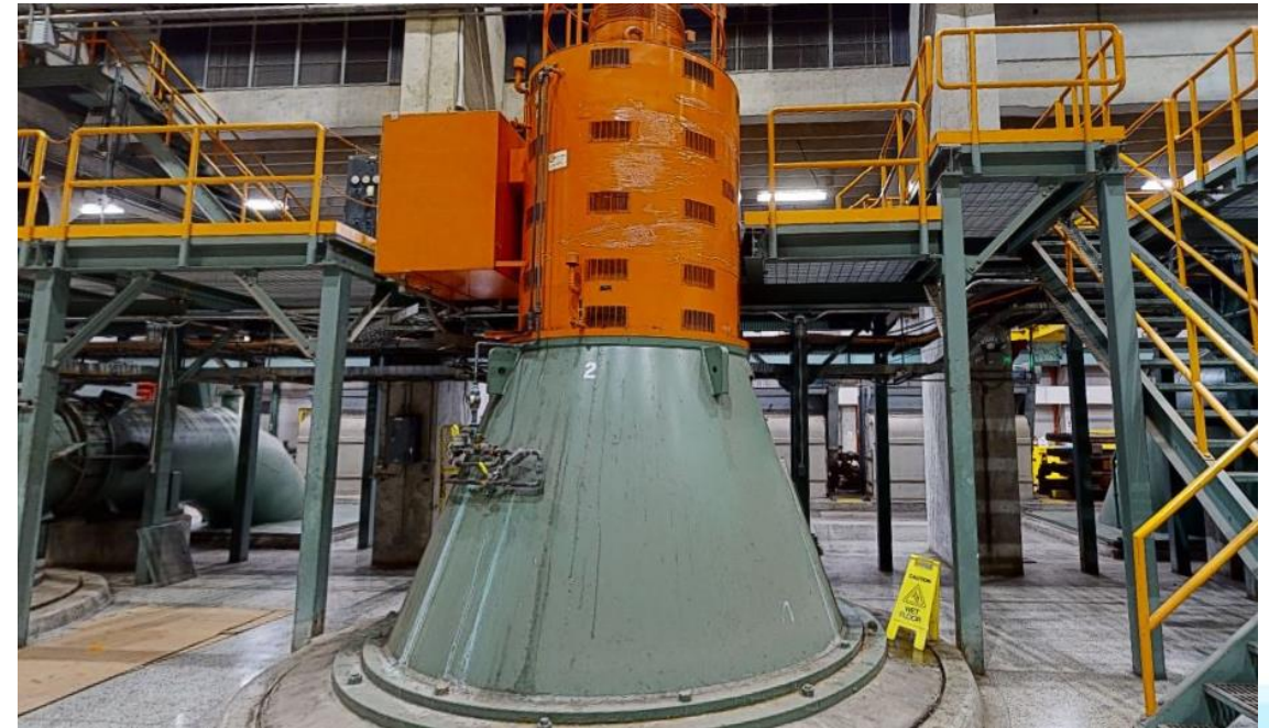
Low Lift Pump 2
