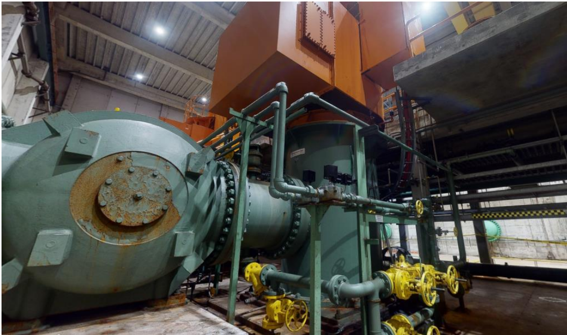
High Lift Pump 8
