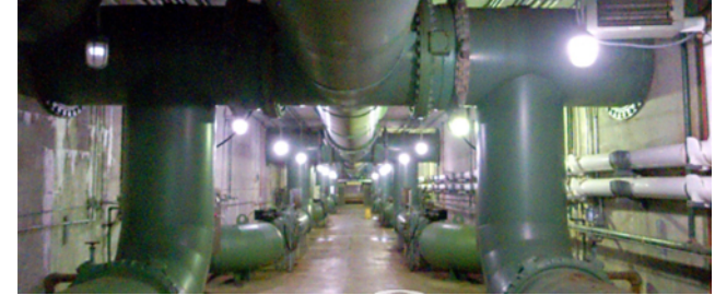
WTP Filtration Improvement
