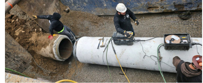
Transmission System Valve
