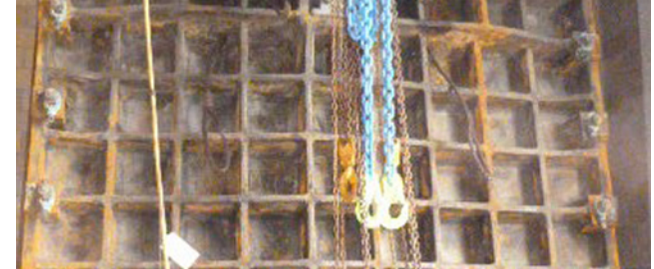
Sedimentation Basin Sluice Gates
