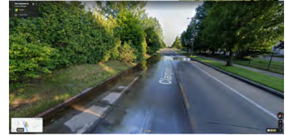
Photo of the berm leaking into Clairpointe
