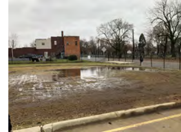
Poor Drainage at Leib
