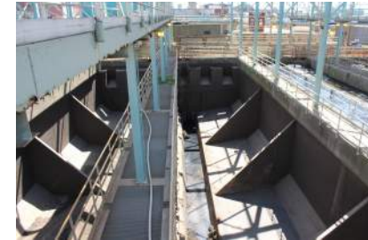
Pump Station 2, Grit channels
