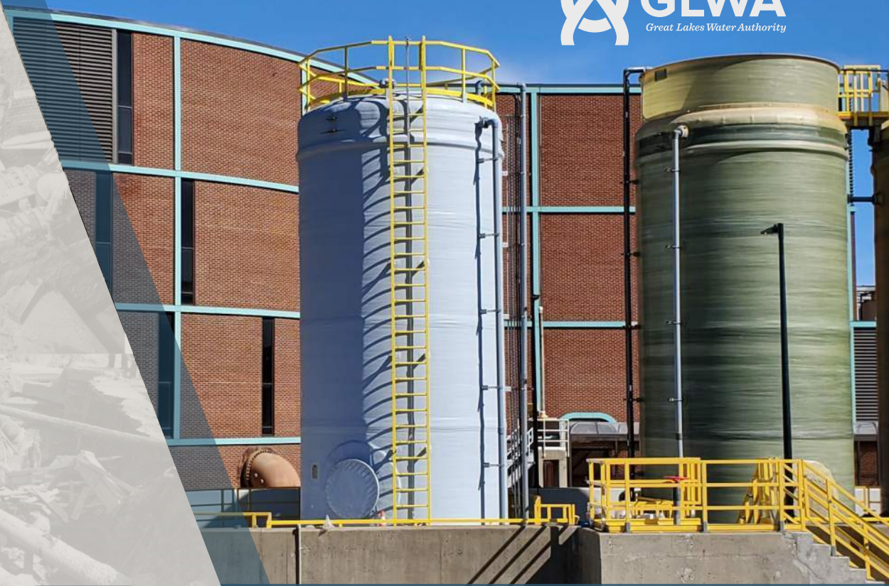
Pump Station 1 Ferric Chloride Storage Tank #3
