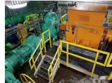
Inside Joy Road Pumping Station
