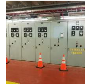
Representative Switchgear to be Replaced under CIP 111001
