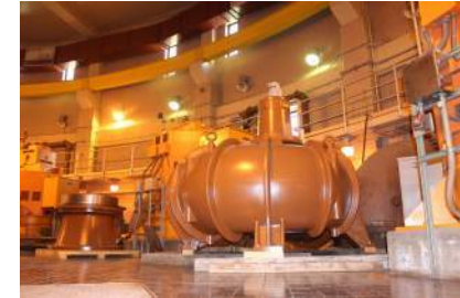
Main Raw Sewage Pumps at Pump Station 2
