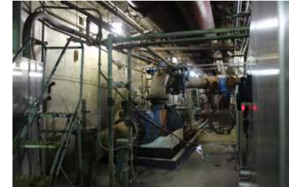
Sludge Feed pump in Complex A
