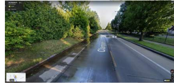
Photo of the berm leaking into Clairpointe
