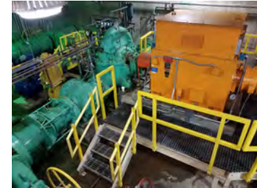
Inside Joy Road Pumping Station
