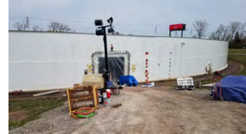
Reservoir No. 3, Access door cut into side of reservoir to perform work.
