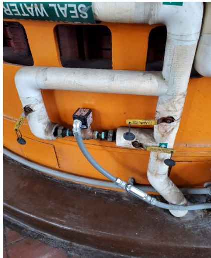
Newly installed solenoid valve will conserve water usage
