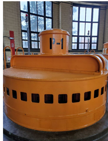
WRRF's Main Lift Pump #1 motor
