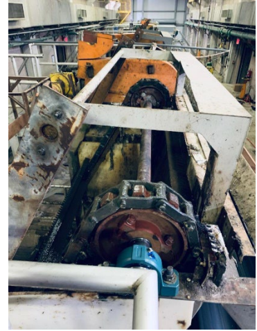
New sprockets and bearings on a bar rack at WRRF's Pump Station 2
