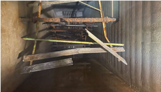
Existing flocculator equipment Sedimentation Basin #1
