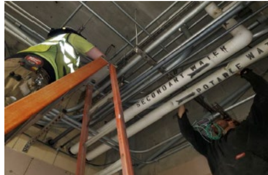
Conduits in Chemical Building
