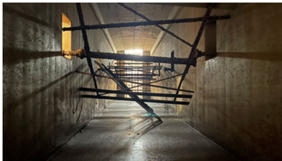
Existing flocculation equipment Sedimentation Basin #4
