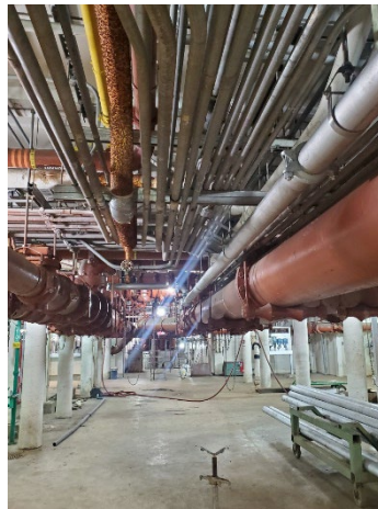
Corroded pipe before replacement
