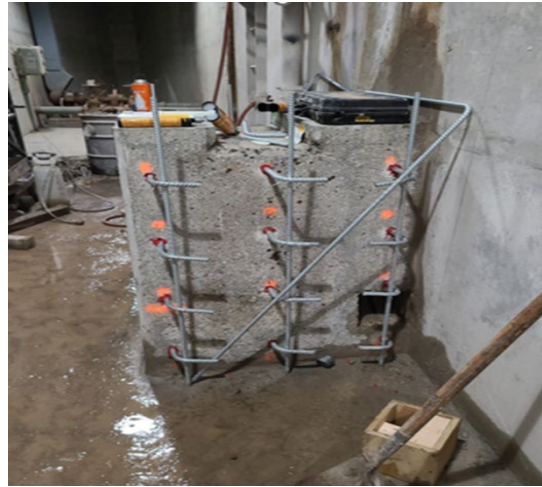
Concrete modifications to existing pedestals for pedestals south drywell (basins #3 and #4) new motors and drives
