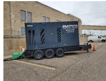
Emergency generator/Low Lift area
