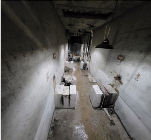
Demolished chain guards, gear, and saw cut concrete pedestals south drywell (basins #3 and #4)
