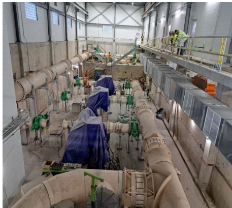
Pump Station 635 pump floor
