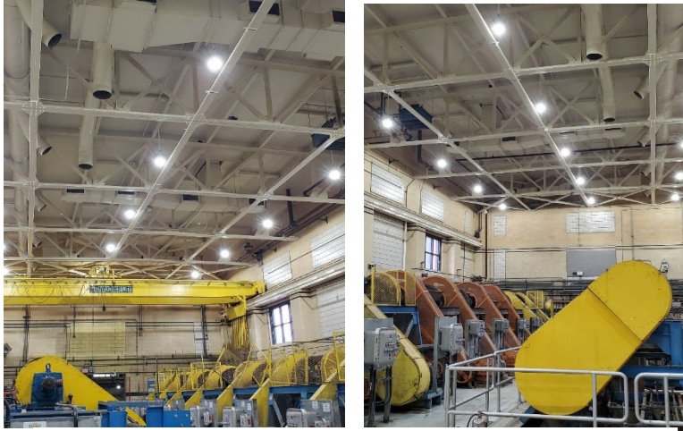
New lighting installed at PSI Rack and Grit dramatically improves conditions for team members
