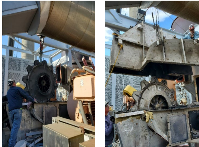
The new impeller for ID Fan 7 is being installed on the roof of Complex II. This job required the use of a 120-ton crane to lift the parts to the roof of the 5-story building
