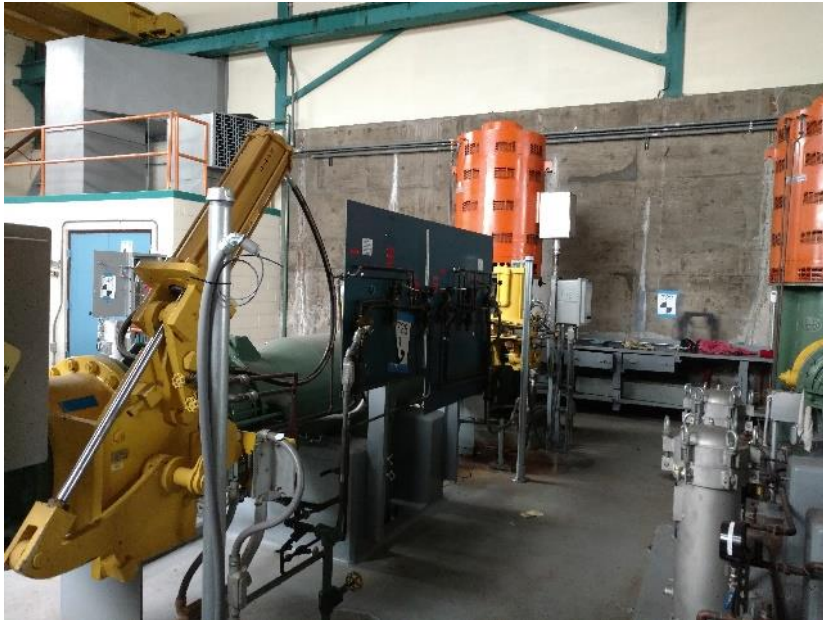
Original Control Butterfly Valves and Hydraulic Control Panels
