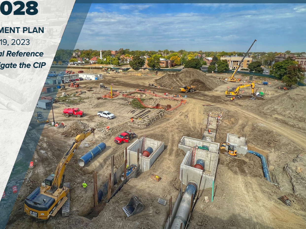
Water Works Park Water Treatment Plant Yard Piping, Valves, and Venturi Meters Replacement Photo submitted by: Jacob Magnum of Water and Field Services
